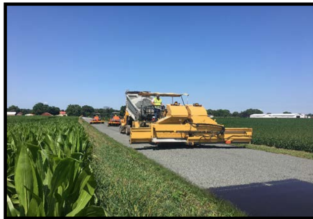
YZ Avenue - Prairie Brook Rd to East Township Line, Prairie Ronde Township
